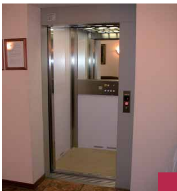
Installation in a hotel (Russia), car with skin plate panels, push buttons and car profiles in stainless steel, half wall mirror.
